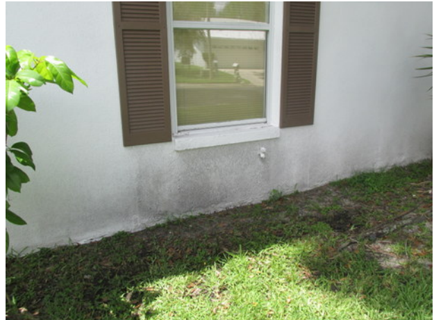
Stucco wall stain
