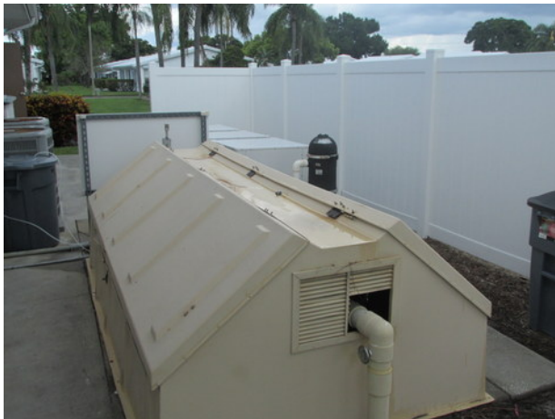
Pool mechanical equipment
