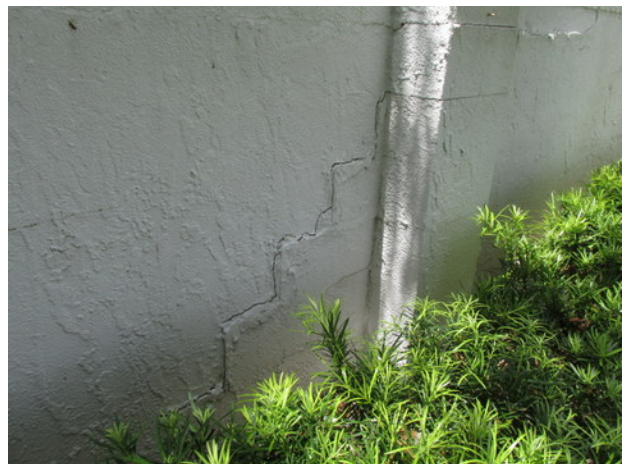
Step cracks at south perimeter wall
