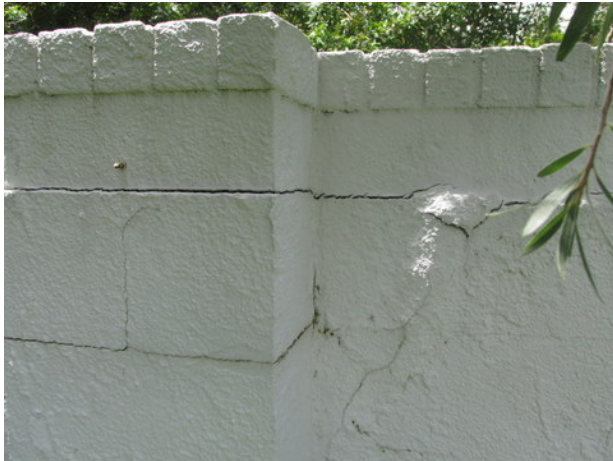
Severe stucco cracks
