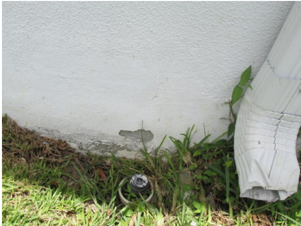
Stucco finish deterioration
