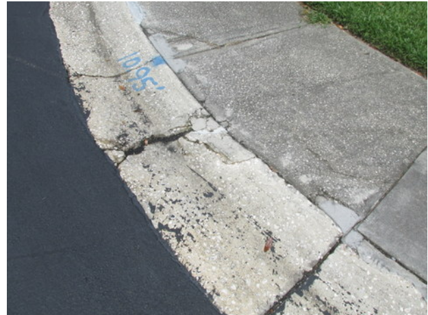
Concrete gutter damage
