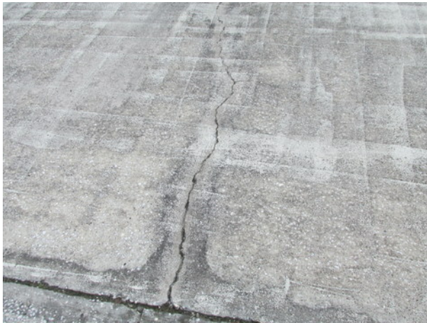
Driveway crack at 9145 37 th Street
