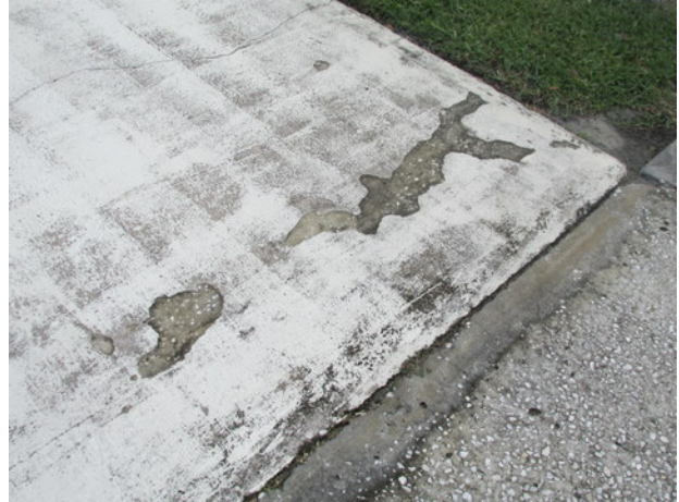
Concrete driveway spalling at 3645 91 st Avenue
