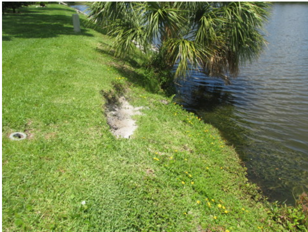
Shoreline erosion at north pond
