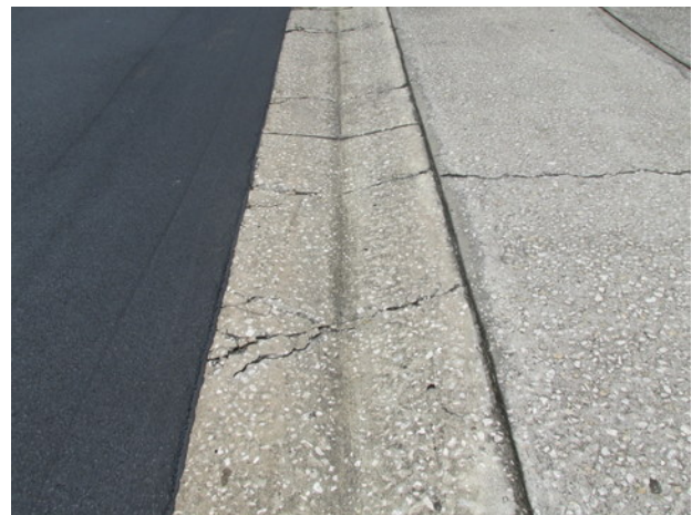
Concrete gutter overview with typical cracks
