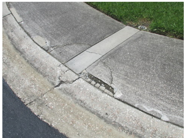
Sidewalk edge deterioration
