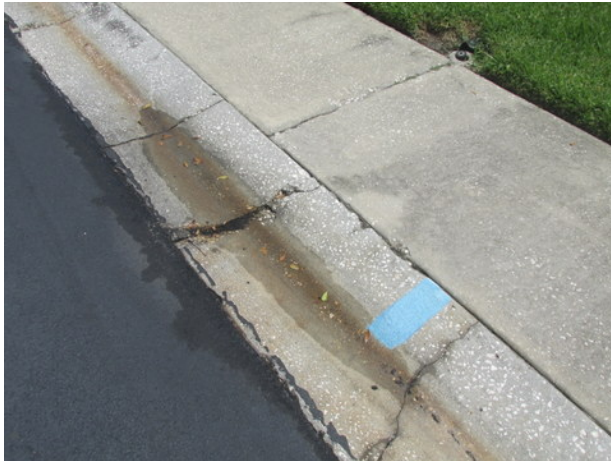
Typical concrete gutter cracks
