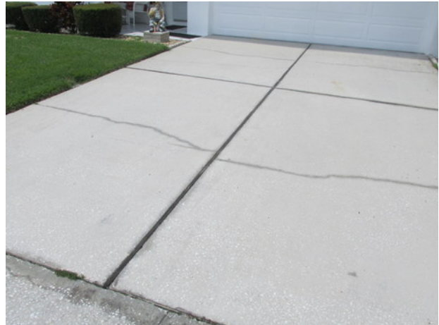
Typical concrete driveway cracks
