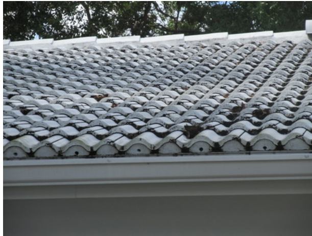
Concrete tile roof with biological growth
