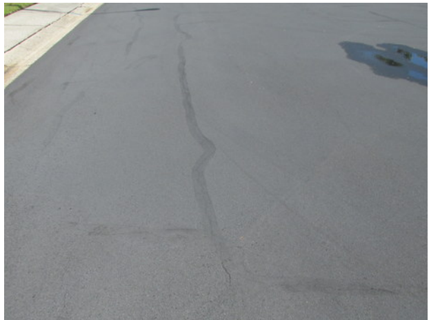
Previous crack repair
