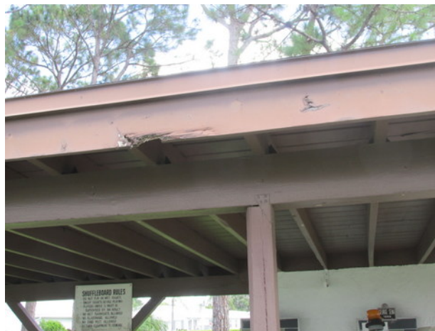
Deteriorated wood components
