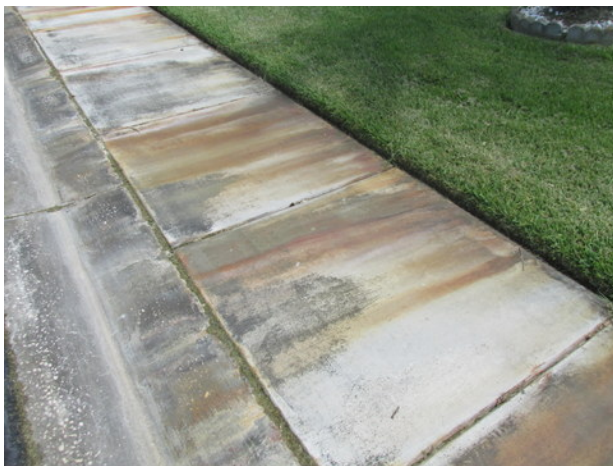
Concrete sidewalk staining
