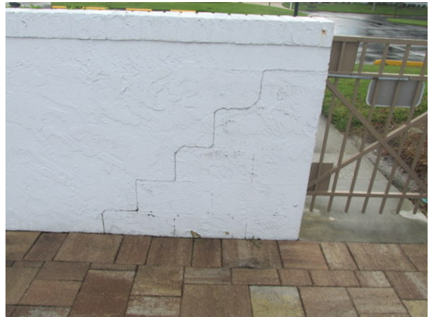
Step cracks at pool perimeter wall
