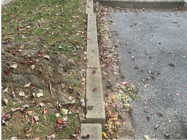
Concrete curb and gutter displacement
