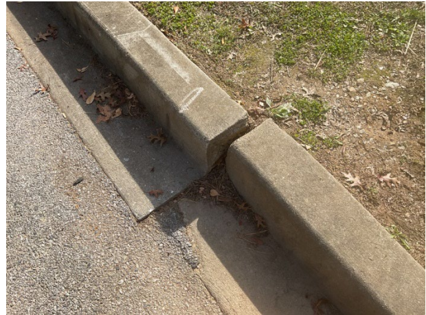
Concrete curb and gutter displacement
