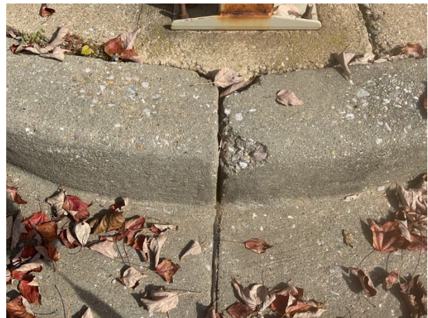
Concrete spall and scaling
