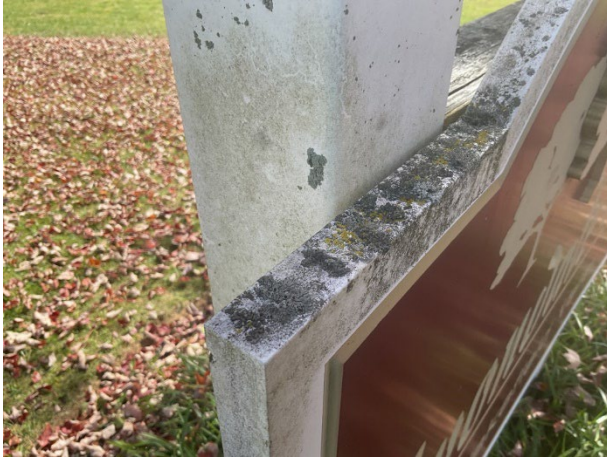
Finish deterioration and organic growth
