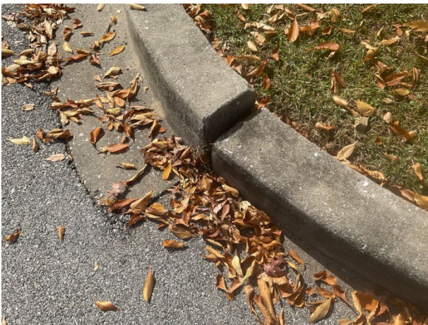
Concrete curb and gutter displacement
