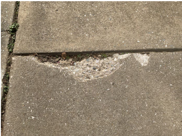
Concrete sidewalk spall
